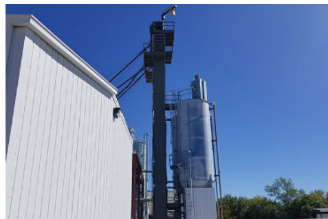
Bucket Elevators Can Sometimes Be Several Hundred Feet Above Ground Level
