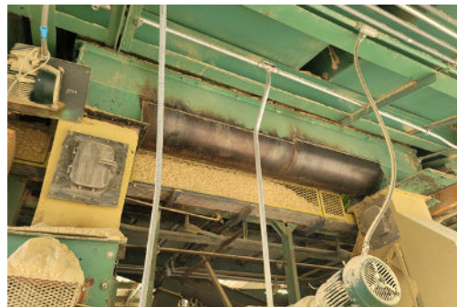
Old Screw Conveyor was Worn Out and Needed Replacement
