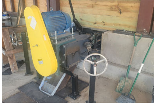
KWS Sized Screw Feeder for Desired Load Out Capacity and Upset Conditions.
